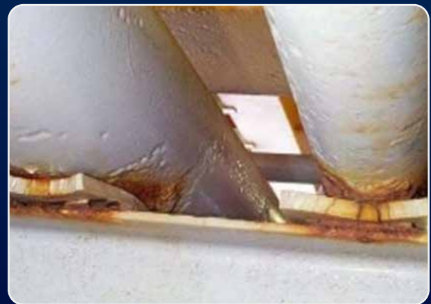
Corrosion Under Pipe Support (CUPS)
