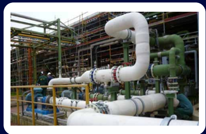
Technical engineering team to designed nonmetallic (FRP and PP/PTFE dual lamination) piping systems.
