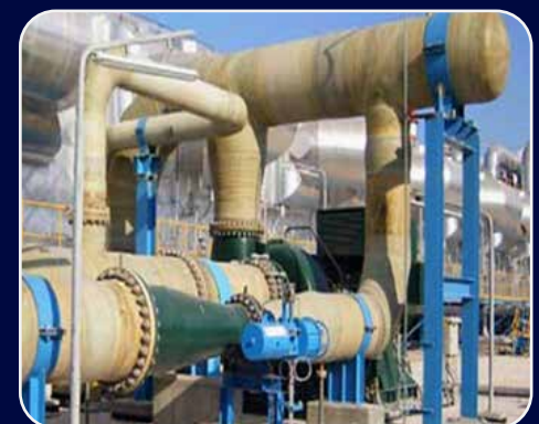
Visual inspection of FRP ,discoloration, Cracks, ultraviolet coating damaged and pipe support inspection
